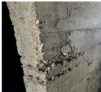
Figure 2.23 demonstrate the segregation in shear wall
