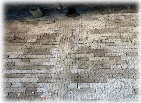
Figure 2.9 concrete juice on the wall before the internal plastering
