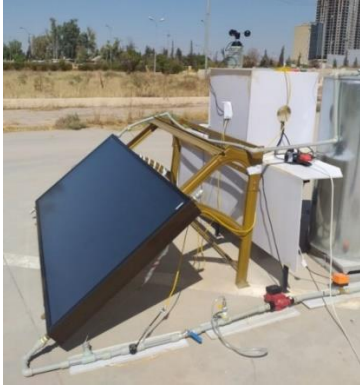
Figure 2. Experimental setup for the water heating solar system
