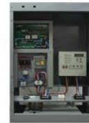
MCF Control Panel
