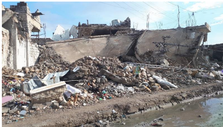
Completely destroyed/ Rehabilitation is not feasible
