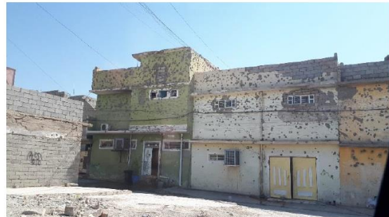
Minor damages to walls, doors and windows
