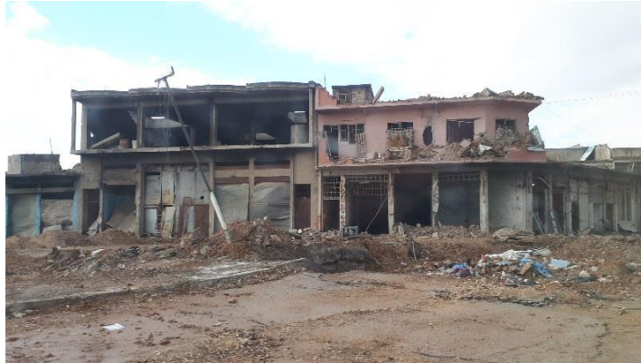
Major damages but structurally not compromised
