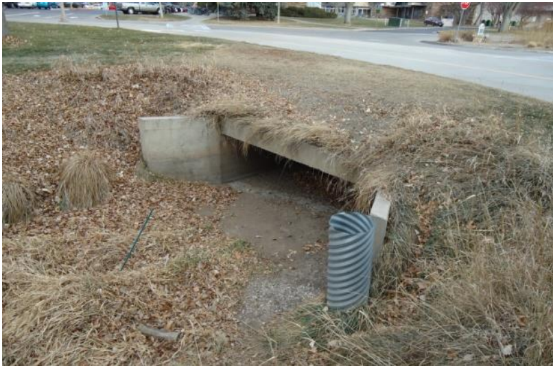
Poor maintenance blocking the culvert drain
