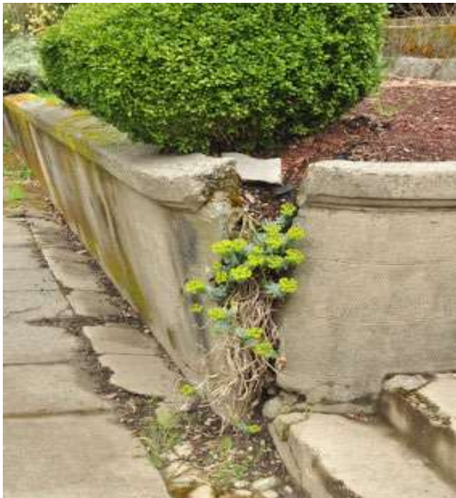
Figure 1.6 Vegetation growth caused to fail of retaining wall
