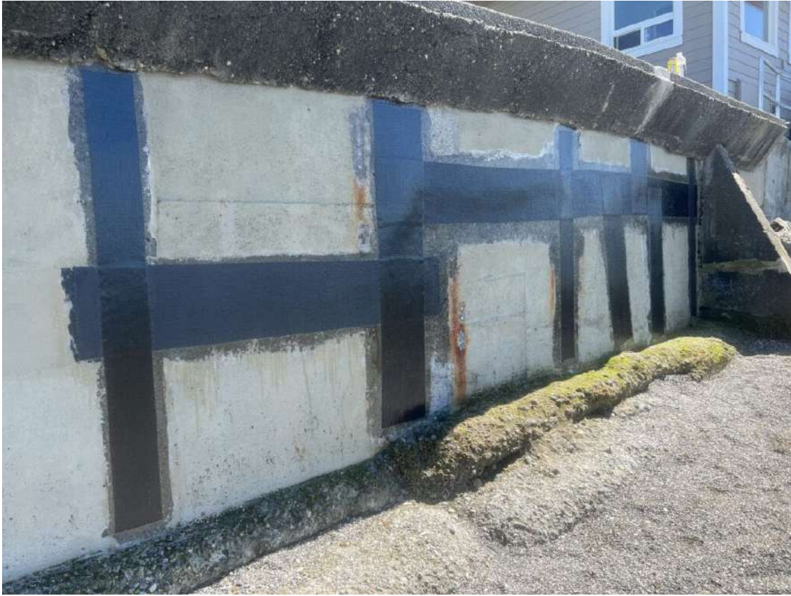
Figure 1.7 retaining wall maintenance properly over time to prevent the fail
