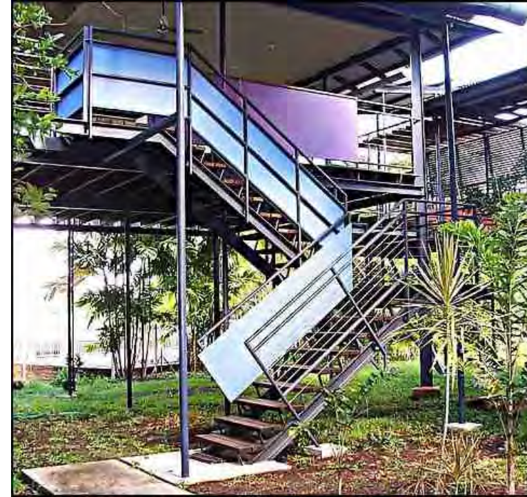
Steel stairs - External stair to a deck, steel structure with timber treads
