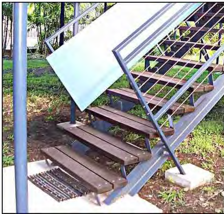
Steel stairs - Bottom of stair concreted in. Note SS wire infills to the handrails one side and fixed FAC panes the other.
