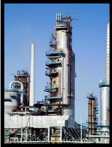
Atmospheric Distillation Tower
